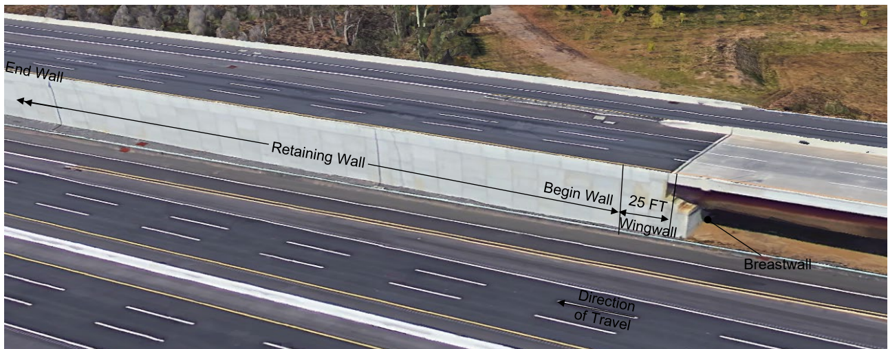
Figure 2-Begin and End of Retaining Wall (No Visible Joint)
