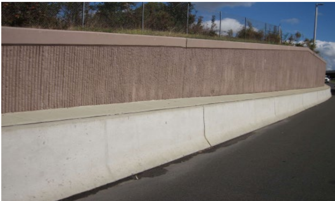
Photo 12 – Other/Combination Wall Steel Sheet Piling with Concrete Facing Retaining Wall (Location – Turnpike Interchange 7 Ramp NOT, MP 53.85NOT)
