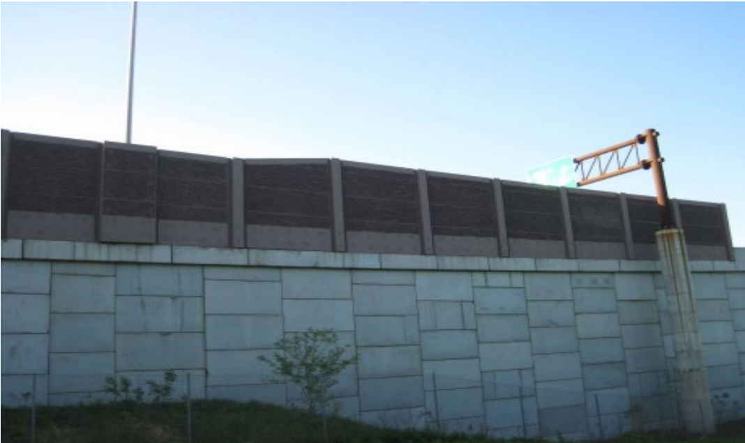
Photo 17 – Other/Combination Noise Barrier Post and Panel Noise Barrier on Top of the MSE Wall (Location – Turnpike NSO, MP 54.00SO SW)
