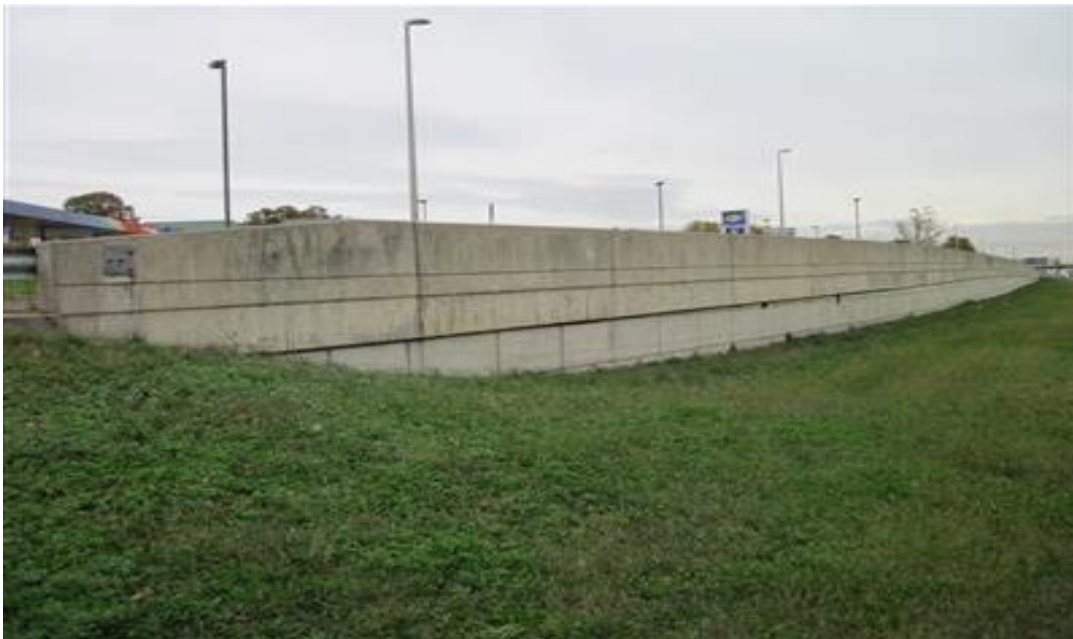
Photo 14 – Other/Combination Wall Prefabricated Modular Wall Panels with Barrier (Location – Turnpike SA7S Ramp SAS, MP 71.72SAS)
