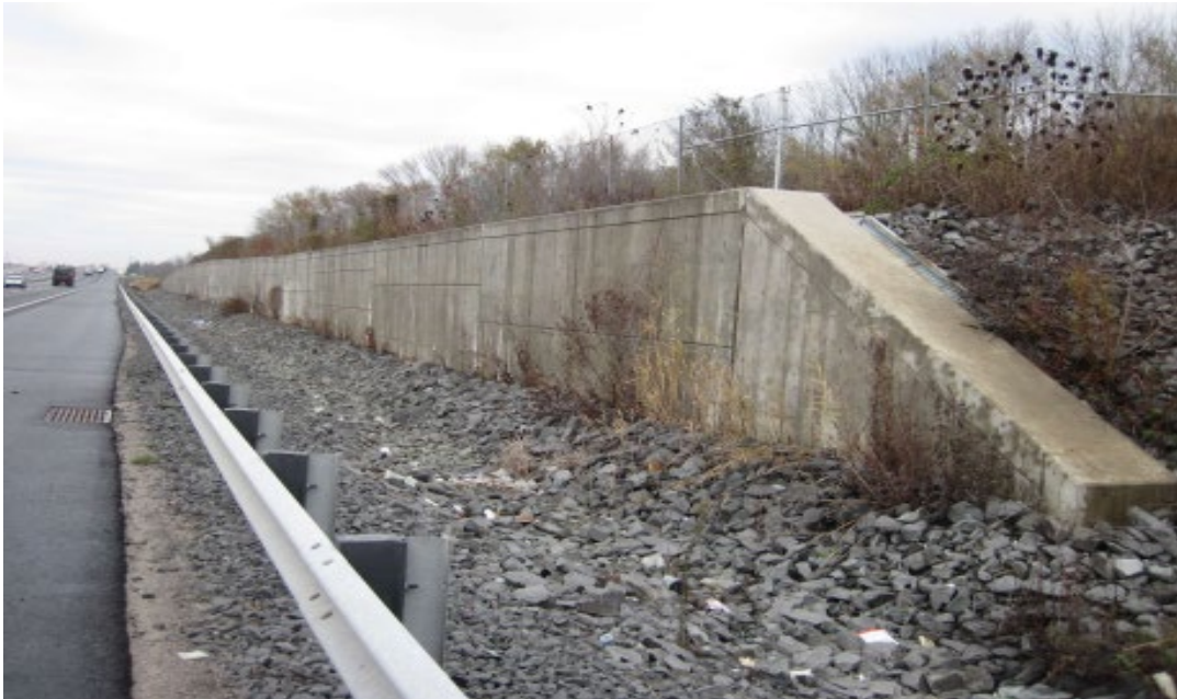
Photo 13 – Other/Combination Wall Timber Lagging with Concrete Facing Retaining Wall (Location – Turnpike NSO, MP 69.3NO)
