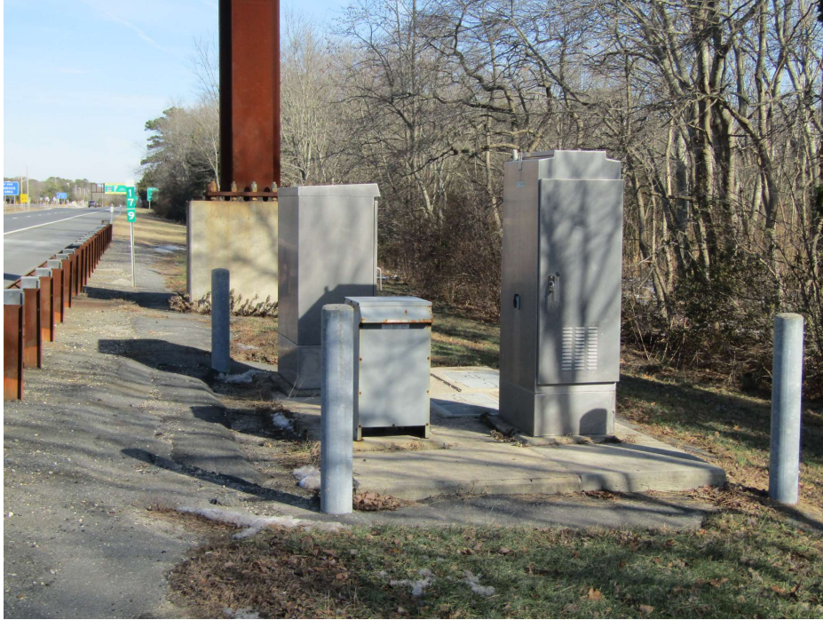
Photograph No. 7 General view of electrical equipment, looking north.
