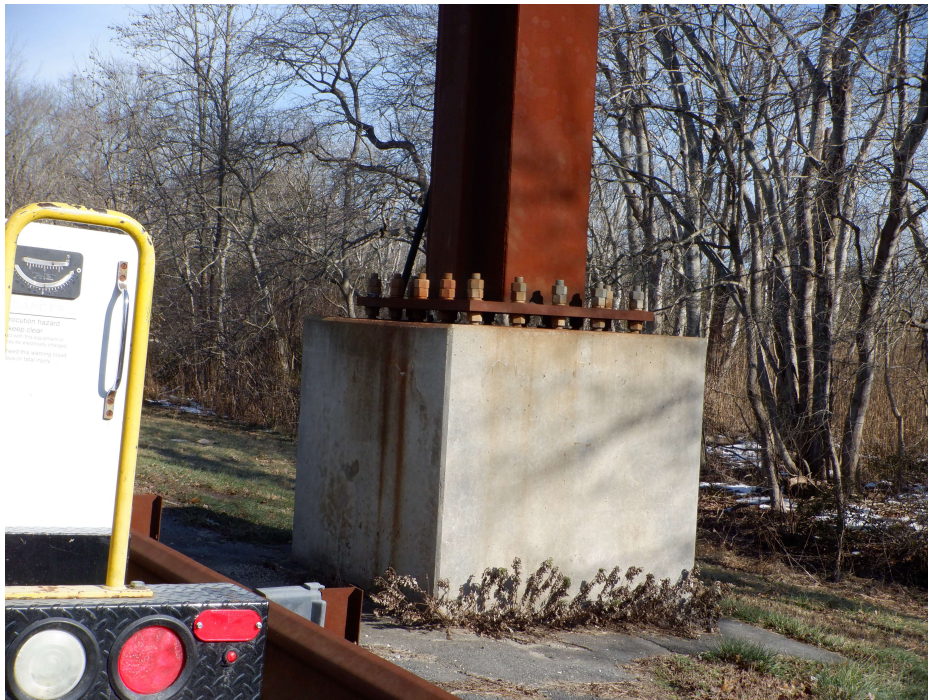
Photograph No. 6 General view of the foundation and base plate, looking northeast.
