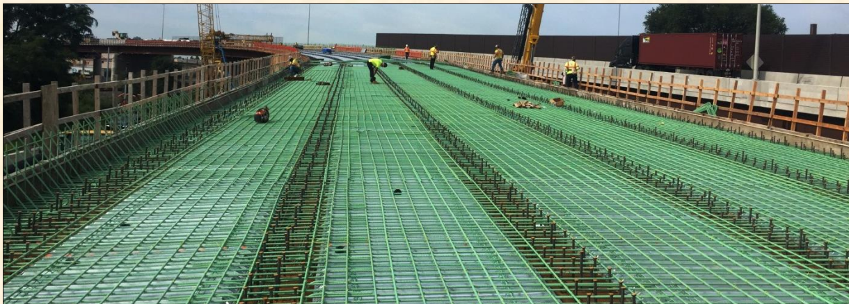
Construction on one of two new bridges being built in connection with the improvements at Interchange 14A
