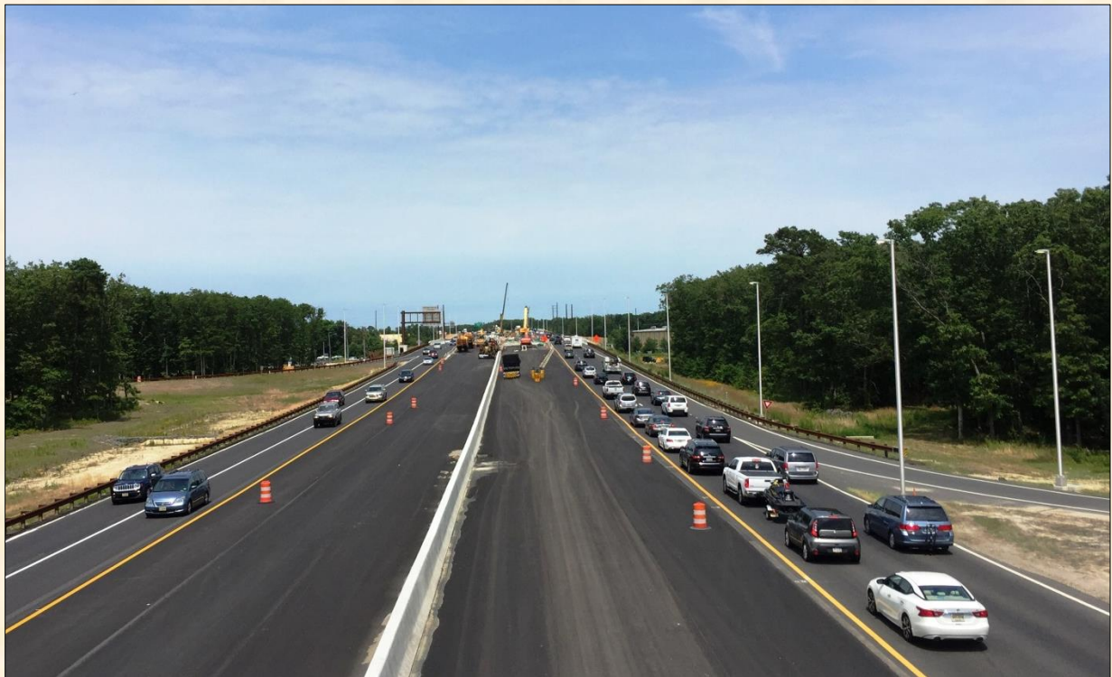
Work on the 3 rd phase of the Garden State Parkway widening, which is scheduled to be finished in 2018
