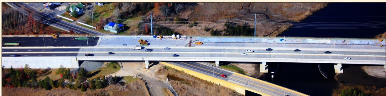
The deck of the Bass River Bridge on the Garden State Parkway was replaced and a new parallel span was built.
