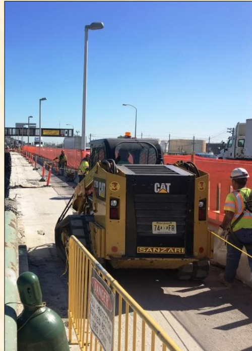
Workers on the westbound side of the NBHCE, just west of the Casciano Bridge
