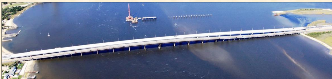
A new Great Egg span was built and one of the existing spans is being rehabilitated.
